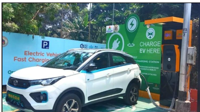
Figure 2 An example of an eco-friendly EV CS in India. This fast-CS in Mumbai is powered entirely by biogas from organic waste, using an on-site biomethane plant to fuel a generator for electricity. It demonstrates how renewable sources can directly replace diesel generators in providing reliable, green power for EVs.
